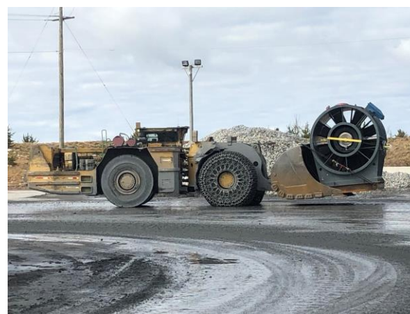
Eagle East main vent fan installation
